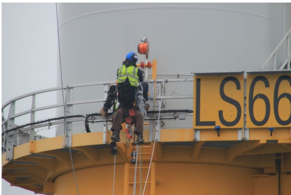
Retrieve ropes from the TP – if required place a deviation on the handrail to prevent any swing
